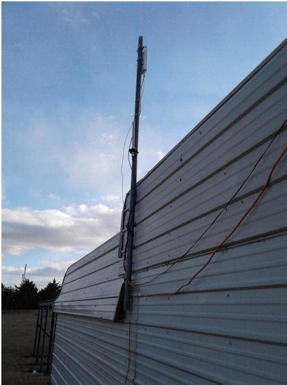
Figure 17: Pole along wall with no over hang.
